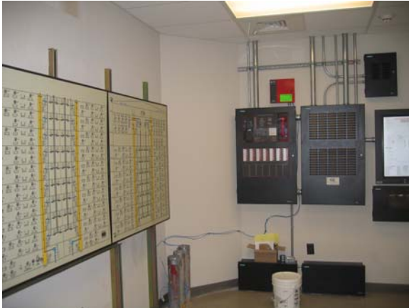
Fig 12 – Fire Command Center
