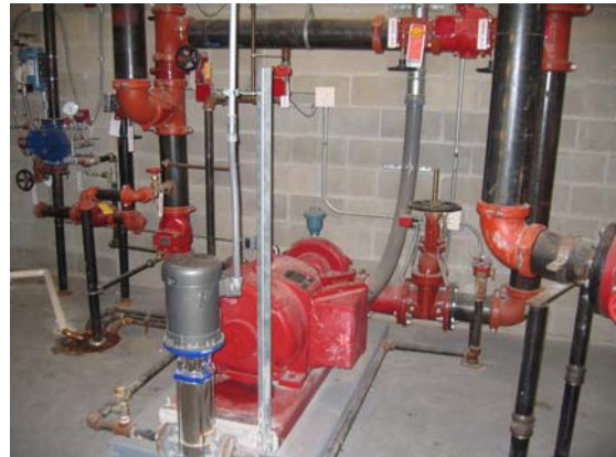
Fig 13 – Fire Pump Room
